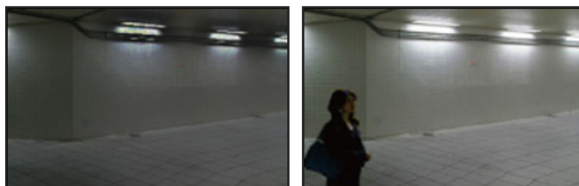
Sensor LED tube light dimmed, conserving energy when no movement is detected (left); Light at full power when movement is detected (right).
